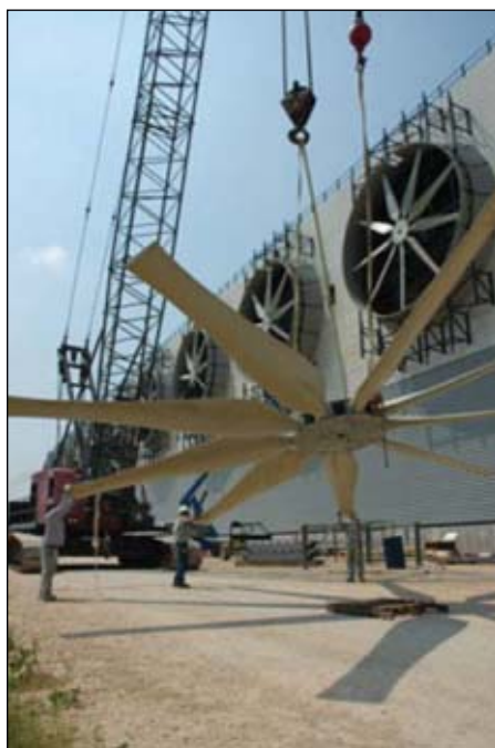
Fan installation proceeds in late 2007 for the ambient-air vaporizers at Freeport LNG. The site will be the first terminal in North America to employ the technology (Fig. 2; photo from Freeport LNG; photo by John Smallwood, Houston).
