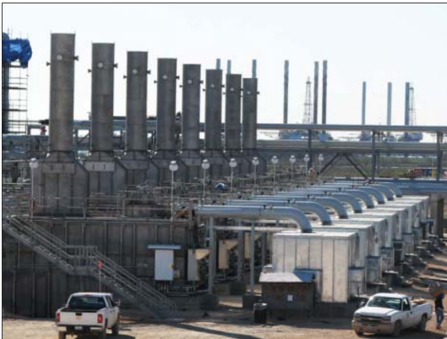
Vaporization at Cheniere's Sabine Pass terminal will be handled by 16 high-pressure submerged combustion vaporizers (Fig. 3; photo from Cheniere LNG).
