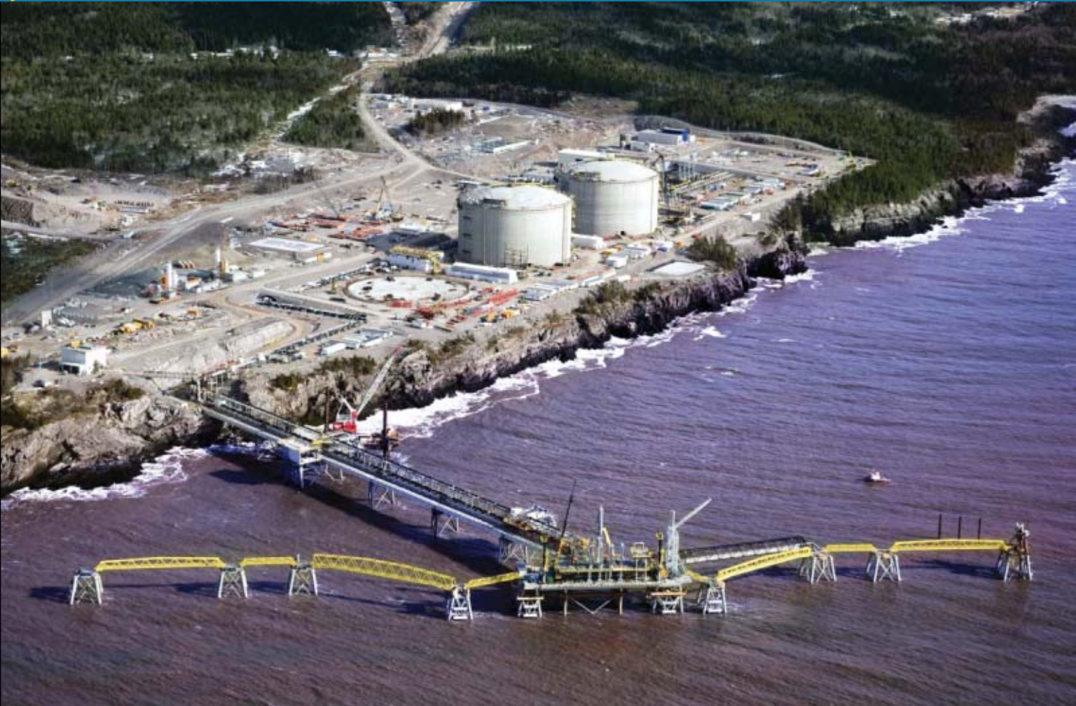
Construction advances at the Canaport LNG receiving and regasification terminal in Saint John, NB. Photo, taken in March, courtesy of Canaport LNG.
